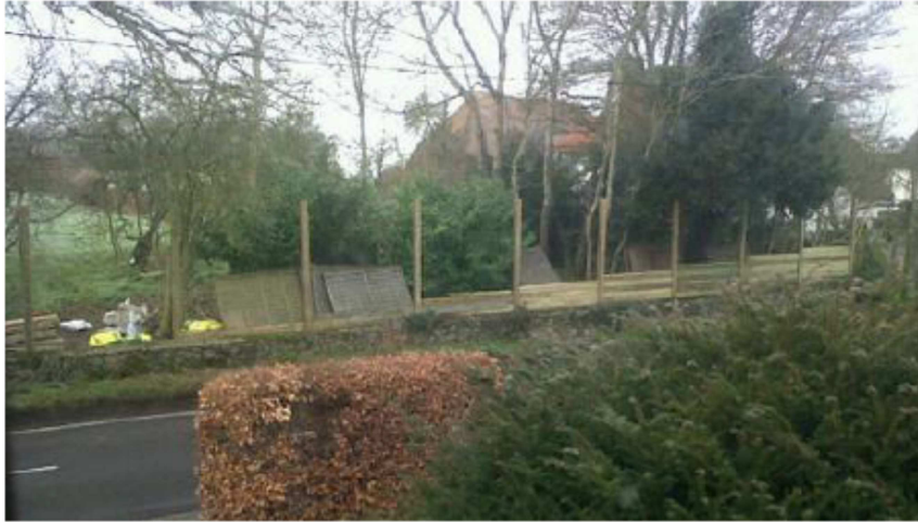
The above photograph was taken during the work and clearly shows the removed panels and the new posts, the difference in height appears to be closer to 1m not 0.4m as stated. Another reference point is the profile of the bushes between the two photographs.
